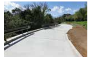
A farm road (Kozushima Village) (Top: before improvement, Bottom: after improvement)
